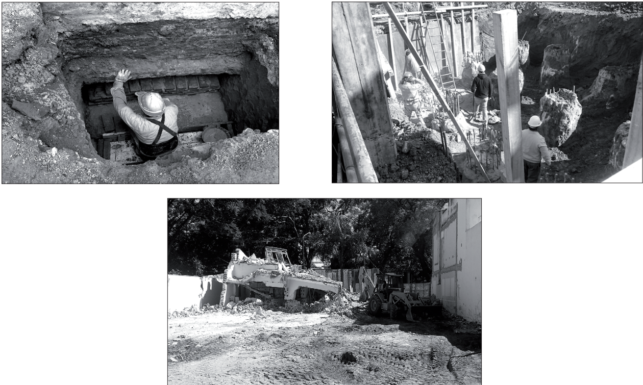
Figure 1 (left): submuring of party walls. Figure 2 (centre): excavation to create subfloors. Figure 3 (right), demolition of existing building. Source: Photographs by the authors.
